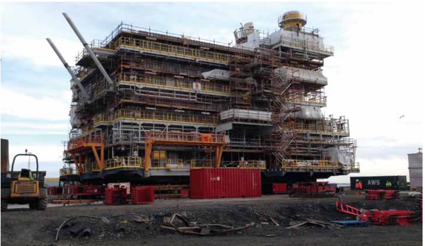
Working directly with Burntisland Fabrications (Bifab), who deliver solutions for offshore energy industries, Lionweld Kennedy supplied steel gratings and welded barrier handrails as a secondary metalwork package for the Cygnus AUQ Topside Platform. The Cygnus field is the largest discovery in the southern North Sea in 25 years, 150km off the coast of Lincolnshire.
