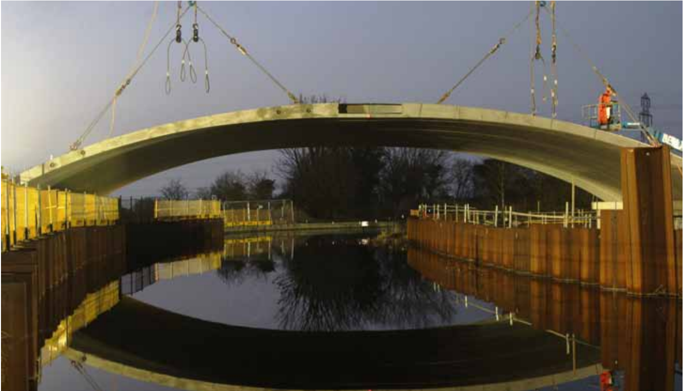
Asset International's BEBO T94 installed on the Heysham to M6 link Milestone Canal Bridge. This is the largest precast over-filled arch constructed in the world.
