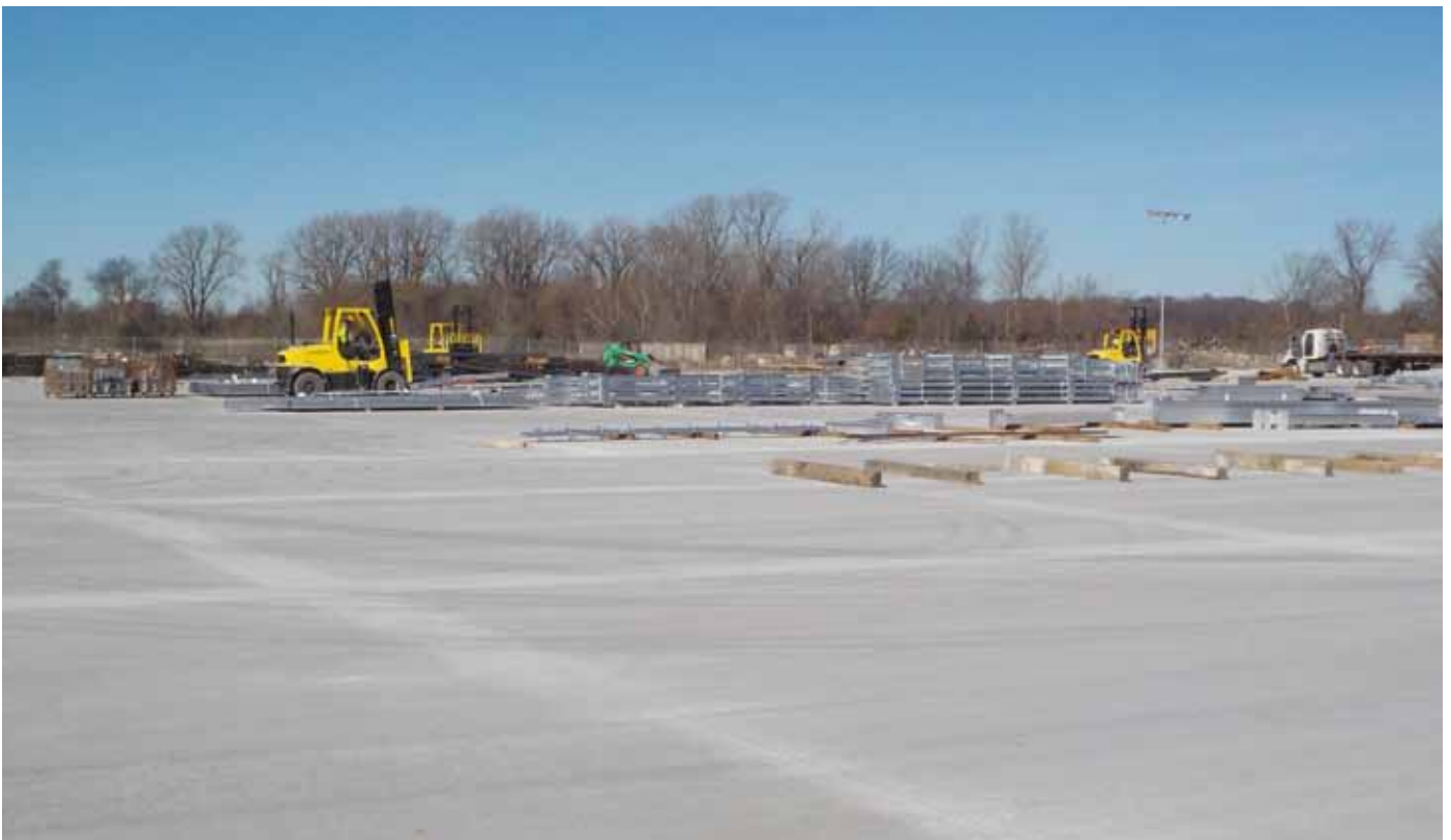
V&S Galvanizing's new plant north of Memphis, Tennessee, USA. The new facility features one of the largest galvanizing kettles in North America.
