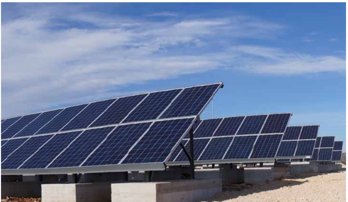
Hill & Smith Solar's 140kw/2 panel rows in a portrait orientation with double leg and concrete ballast foundation, situated in Grude, Bosnia and Herzegovina.
