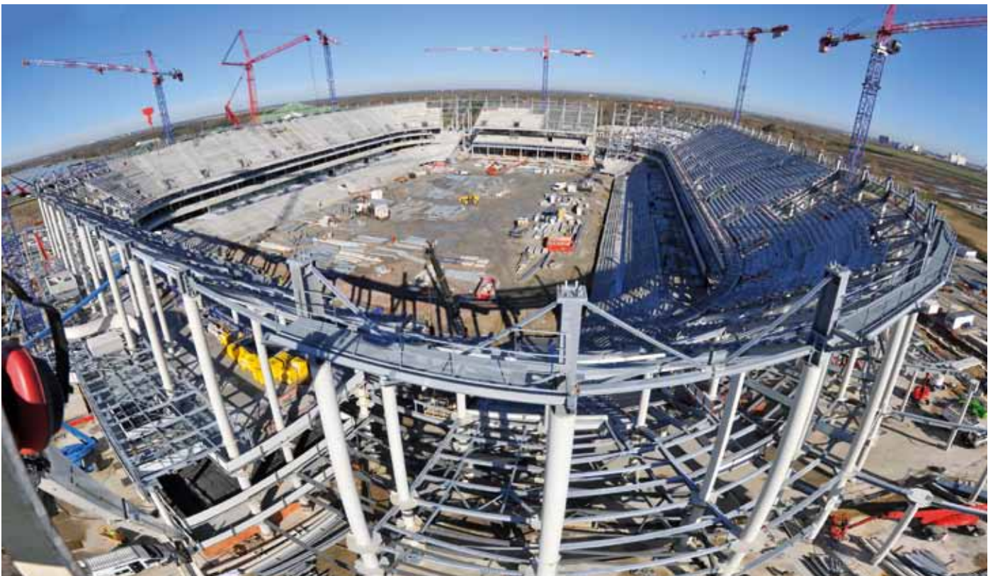
France Galva were given the job of galvanizing the metal framework for the new Bordeaux stadium, France and supplied product during 2013 and the early part of 2014. The stadium, which is due to be finished in April 2015, has a capacity of 43,000 seats, will be the new home of FC Girondins de Bordeaux and is set to host 5 matches of the UEFA Euro 2016.
