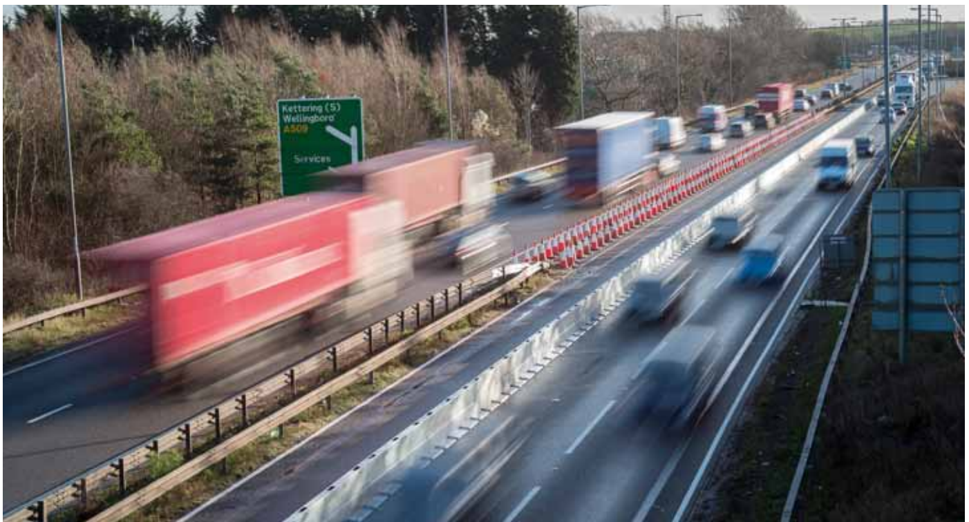
Asset Zoneguard on A14 Morgan Sindall contra flow works N2 W2 system.
