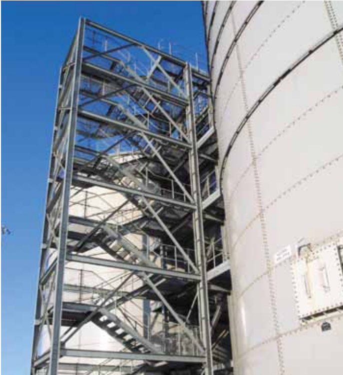
Design fabrication and installation of a multi-flight staircase to the digester tanks for the Mogden sewage treatment works.
