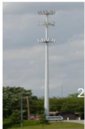
Antenna Tower Pole
